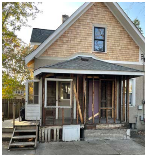
Mid-deconstruction work at the Wilson home, before and after. (Photos supplied by James Wilson)
