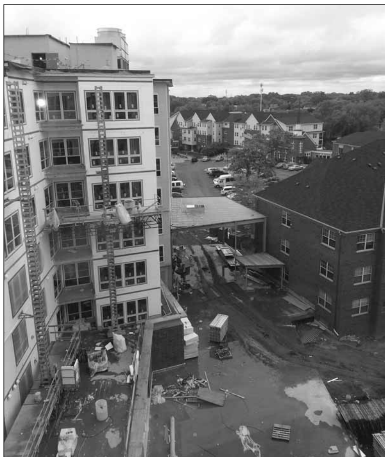
The Terrace, Phase 1 of Midway Village, is being constructed at the corner of University and E. Lynnhurst Ave., and will open in the fall. Paul Hagen, communications director for Episcopal Homes, who is building the project, said that the Green Line coming and Porky's leaving was, "a massive dose of synchronicity." (Photo by Denis Woulfe)
