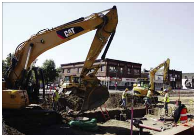
How construction will be staged and monitored has been discussed at numerous meetings between business leaders, University of Minnesota officials, local elected officials and Central Corridor project staff. (Photo by Stefanie Berres)
