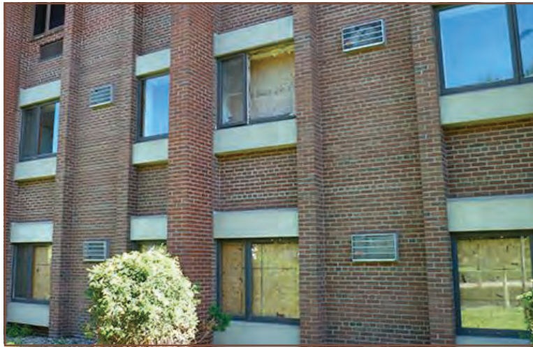
Neighbors say they routinely observe scrapping, squatting, drug sales, and other unwelcome activity in and around the abandoned Midway Pkwy. property that used to be the Sholom Home. (Photo submitted)
