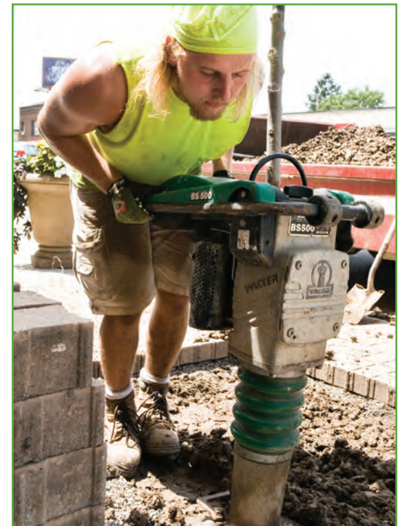
Kyle Hunter compacted the structural soil to hold a new tree in place —while still allowing for good water flow.
