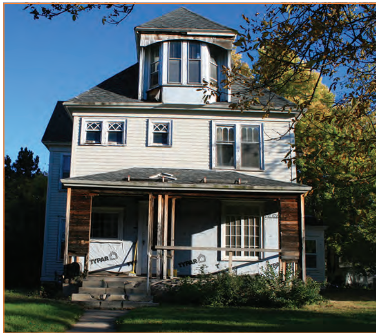
The house at 1549 Minnehaha Ave. dates from 1888 and was home to Prof. W.D. Walcott. He chaired the Hamline University philosophy and psychology department. Demolition was halted in 2014 after the neighborhood raised red flags about its possible destruction. (File photo)
