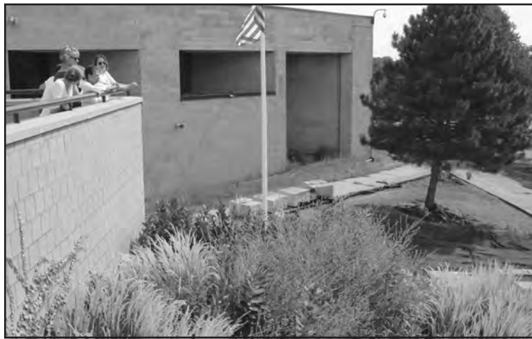
Members of the Transforming Central Committee and Principal Mary Mackbee survey the work being done to create the outdoor classroom in August 2016. "I'm super excited for the outdoor classroom and learning opportunities that the project is installing," said senior Olive Murdoch Meyer, who is the co-president of Roots and Shoots. (Photo by Tesha M. Christensen)
