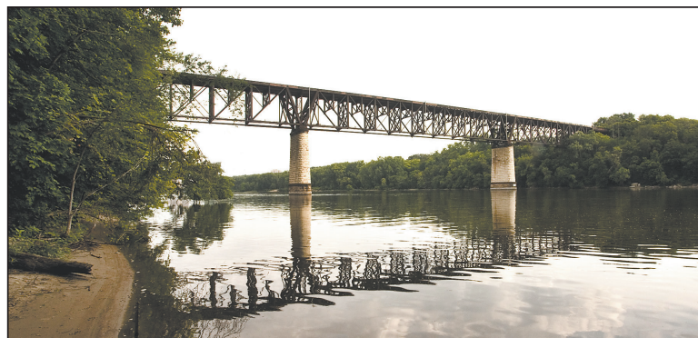
What would it take to make the Short Line RR Bridge east of 27th St. on West River Parkway structurally sound so that it could continue the Midtown Greenway trail across the Mississippi River from Minneapolis into St. Paul? (Photo by Margie O'Loughlin)
