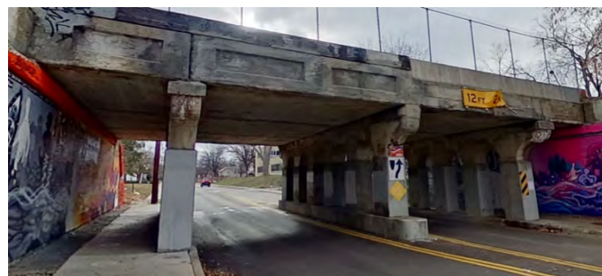
The bridge as it looked after Phase 1 but before Phase 2. (Photo submitted)
