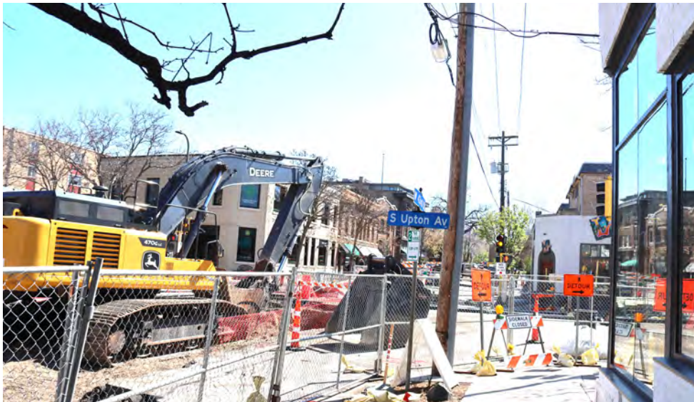
A water line and a sanitary sewer line that are over 100 years old are being replaced at Upton and 43rd, closing the intersection for 10 weeks. (Photo by Tesha M. Christensen)
