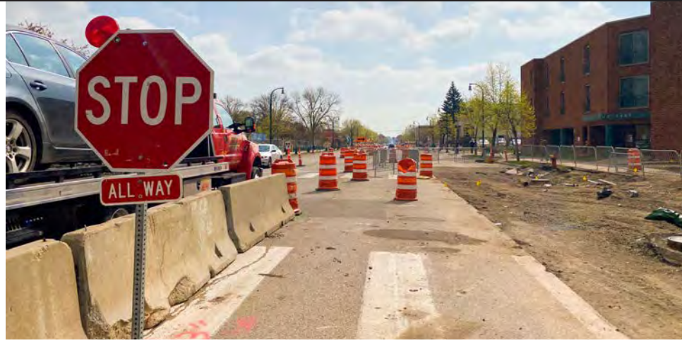
E. Lake Street is torn up in front of the East Lake Library, as work begins on new Bus Rapid Transit stations. Work will primarily be done on the route east of Hiawatha into St. Paul this year, and west of Hiawatha next year. (Photo by Tesha M. Christensen)
