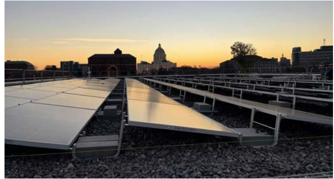
The new St. Paul City School is partially powered by solar panels on the roof.
