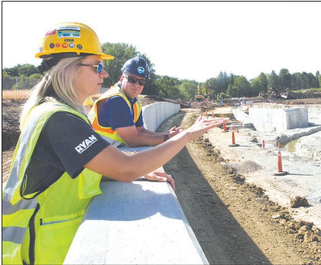
Ryan Companies Parks and Public Spaces project manager Mac Pegovac and Bob Fossum of CRWD check out the progress of the storm water management at the heart of the redevelopment project at the former Ford Assembly Plant property. (Photo by Margie O'Loughlin)
