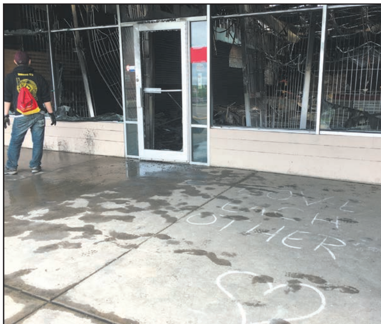
The center of the Midway Shopping Center was the most severely damaged by the fire on May 28, 2020. The shopping center remains vacant and boarded, with a fence around it, more than a year after the damage. (Photo by Tesha M. Christensen)
