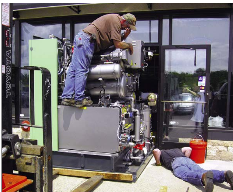
It was a really tight squeeze to get the new equipment through the door of U.S. Cleaners. (Photos by Jan Willms)
