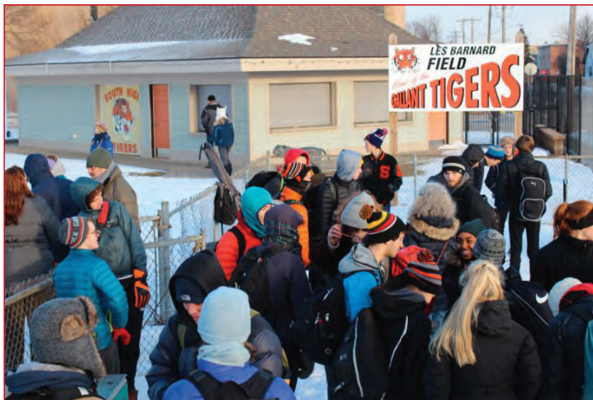
About 100 people stood in bone-chilling temperatures in January 2017 on South High's Barnard Field to rally for fixes to the deteriorating field. According to Emma Schluter, the field isn't safe for either soccer or track and field, the two sports she plays. (Photo submitted)
