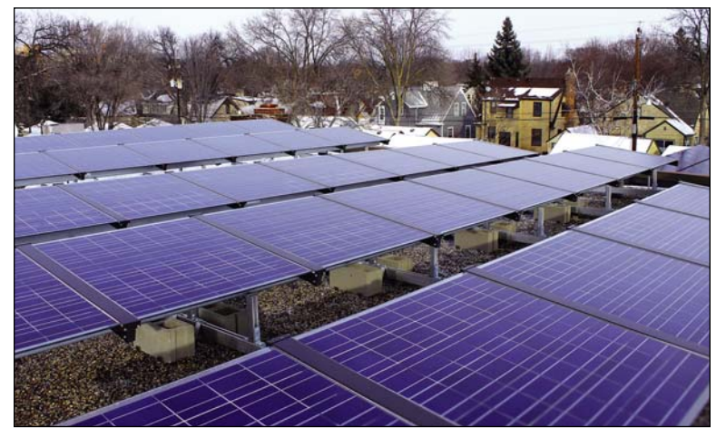
The solar panel array on top of Nokomis True Value Hardware. These panels, along with some panels on top of their storage building, generate up to 17,000 kWh per year.
