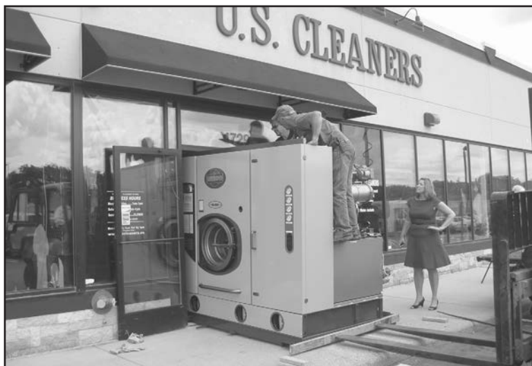
It was a really tight fit last year as U.S. Cleaners moved the new equipment into their location. They have now received a Green Business Award from the city of Minneapolis. (Photo by Jan Willms)
