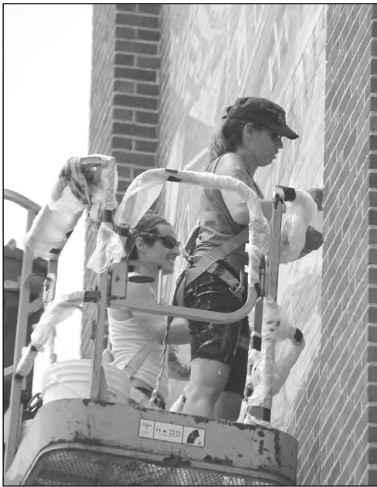
Project manager Claudia Valentino (right) and Bernardo Reyes work to install the mural on the wall on Wed., July 15. "The people who get to look at it every day got to be a part of it," remarked Reyes. (Photo by Tesha M. Christensen)
