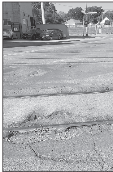
Here is a before photo showing the potholes and damage to the surface of 33rd. (Photo submitted)
