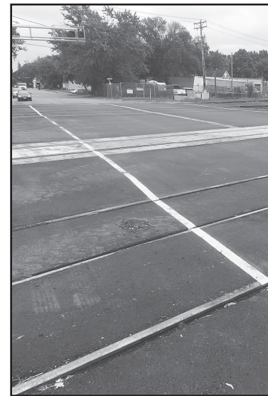
A new surface means a smoother ride for those traveling over the tracks. (Photo by Tesha M. Christensen)
