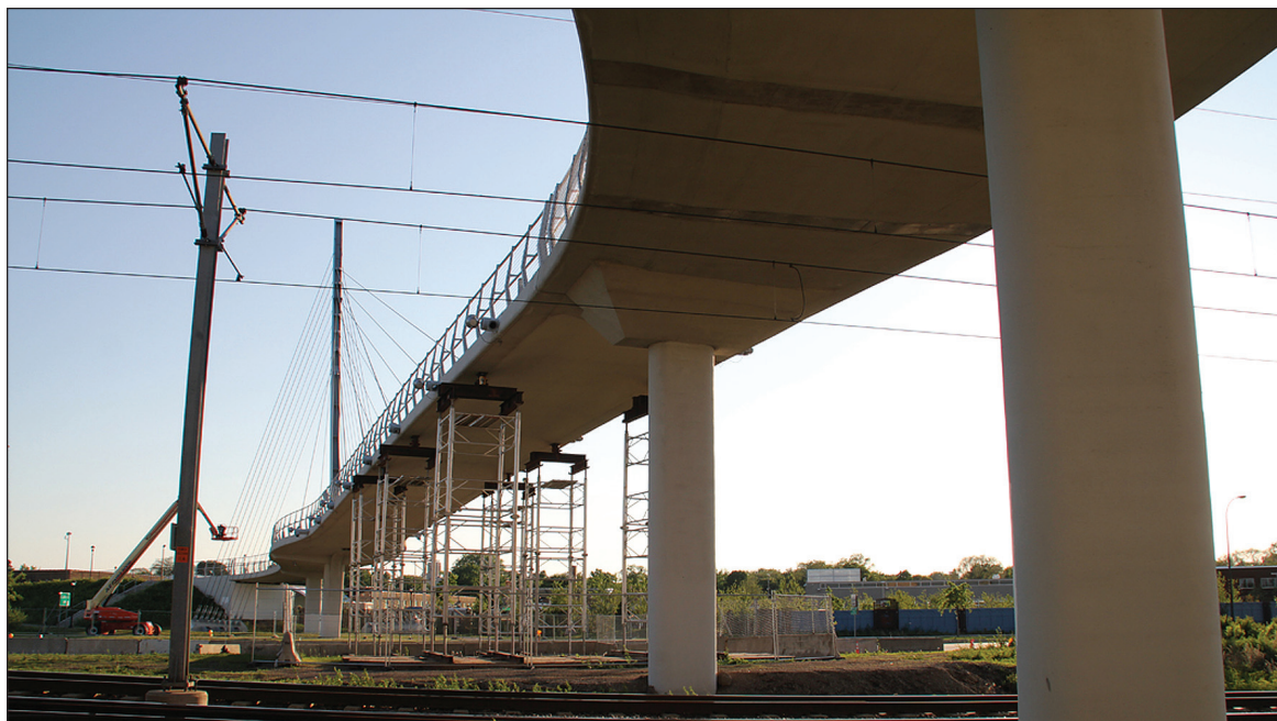
The Sabo Bridge was closed on February 20, when two of the cables that support the bridge fell due to cracks in their attachment points; additional significant cracks were subsequently found in two other support plates. (Photo by Tesha M. Christensen)
