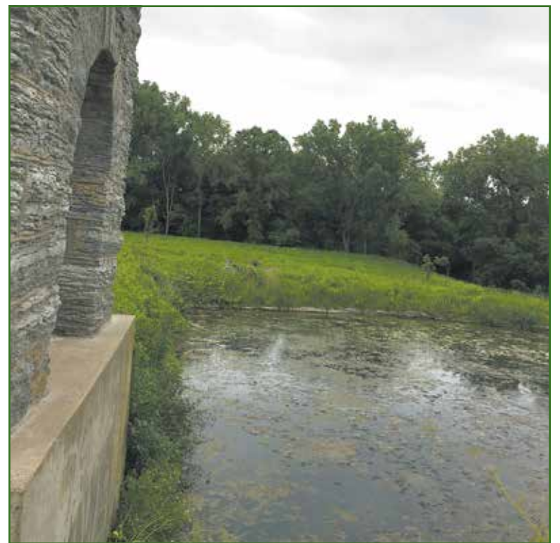
A sewer tunnel project near 3901 Minnehaha Parkway E. may affect the flow of water at Coldwater Spring, but the Metropolitan Council Environmental Services (MCES) is working to minimize the impact. (Photo by Tesha M. Christensen)
