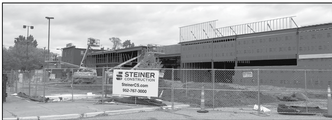
Work is now underway renovating the west side of the former Rainbow Foods building for Aldi and the adjacent retail. The entire west facade will be replaced. Various pedestrian improvements will be made adjacent to the new retail entrances including new sidewalks, a raised pedestrian crossing connecting Aldi to the parking lot, plantings and bike racks. (Photo by Tesha M. Christensen)
