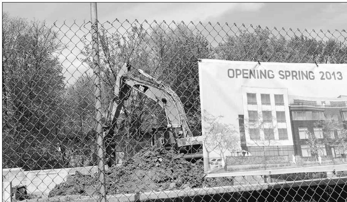
In place of a 32 unit condominium, developer Michael Lander is building a 48 unit apartment building at the 46th Street site. The apartments will be built on the foundation that had been laid for the earlier development. (Photo by Stefanie Berres)
