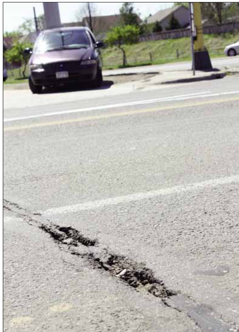
According to City Council Member Gary Schiff, the city of Minneapolis has been asking Soo Line/MN Commercial Rail to repair the broken pavement and railroad ties on E. 35th St. just east of Hiawatha, for the past 10 years. (Photo by Stefanie Berres)
