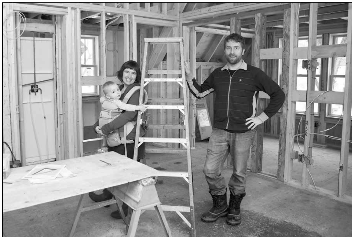
Stephanie Erickson, Ross Pfund and baby Quinlan in their partially completed accessory dwelling unit. The new structure will have a living room, kitchenette, ¾ bathroom and bedroom over a double garage. A forced air furnace is located under the interior staircase. (Photo by Margie O'Loughlin)
