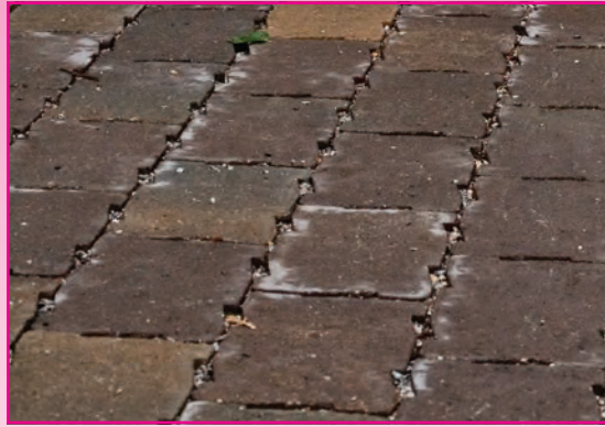
Photo above: Pervious pavers are a much more environmentally friendly choice than asphalt or concrete. Water is allowed to penetrate into the ground between pavers, which decreases run-off into Lake Nokomis. Pervious pavers may be installed as a buffer between where the driveway meets the alley.
