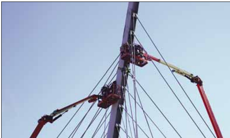
Crews work to install and retrofit diaphragm plates on the Sabo Bridge pylon. The bridge was closed in October and will not reopen to pedestrian and bicycle traffic until work is completed in early December. (Photo by Tessa M. Christensen)
