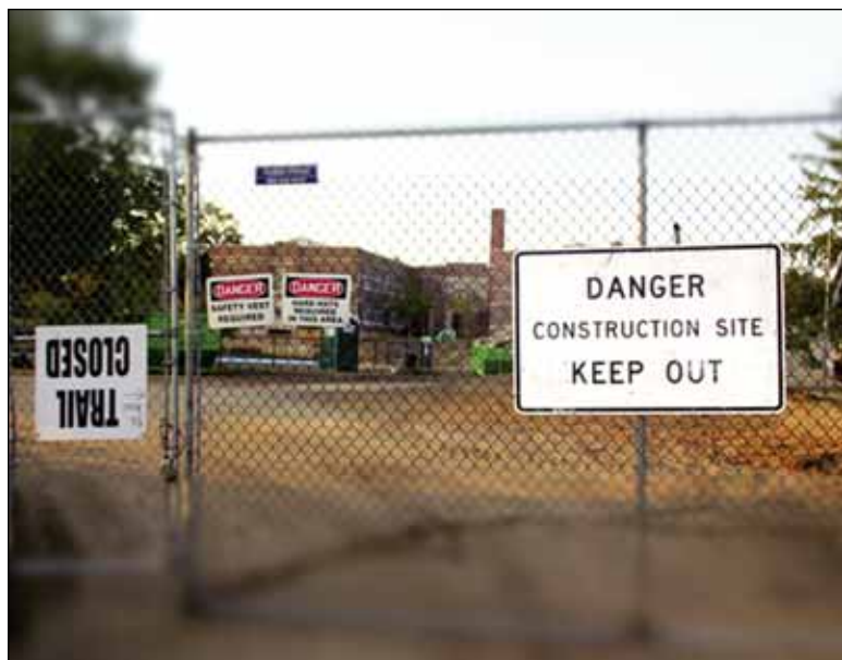
Construction continues on Keewaydin School. A fence near the Rec Center keeps people out of the construction site. Work will be complete in time for the start of the 2013-14 school year. The wading pool and playground equipment currently in place will remain there for about five years to give the park board time to create a new playground on the southeast corner of their property. (Photo by Tesha M. Christensen)
