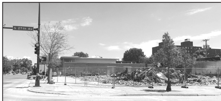
The Oddfellows/El Nuevo Rodeo building at E. Lake St. and 27th, where both George Floyd and former Minneapolis Police Officer Derek Chauvin worked, has been demolished. Community leaders are talking about how to hold sites for local development and small businesses versus purchase by outside investors. (Photo by Tesha M. Christensen)
