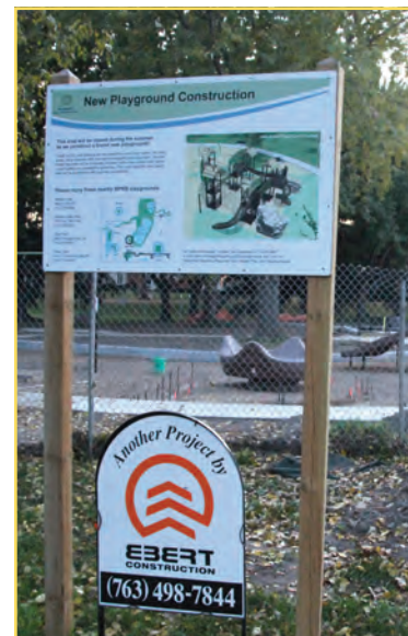
Neighbors have questioned why the playground equipment has been sitting there since June but children haven't been able to play there. The answer is that MPRB bid the equipment and surfacing separately, racing to meet grant fund deadlines. (Photo by Tesha M. Christensen)
