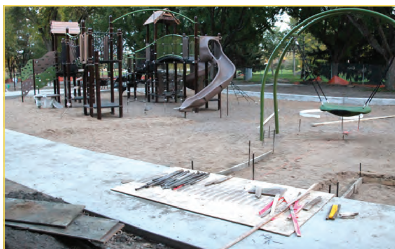
Rain has delayed work this fall on the concrete and asphalt trails, as well as the playground surfacing, at Triangle Park. According to MPRB Commissioner Steffanie Musich, weather delays may prohibit this project's completion this fall. Temporary fill options and ways of curing the pour-in-place surfaces under play equipment are being explored. If not completed this fall, remaining work will be done in 2016 when ground conditions and temperatures meet material requirements. (Photo by Tesha M. Christensen)
