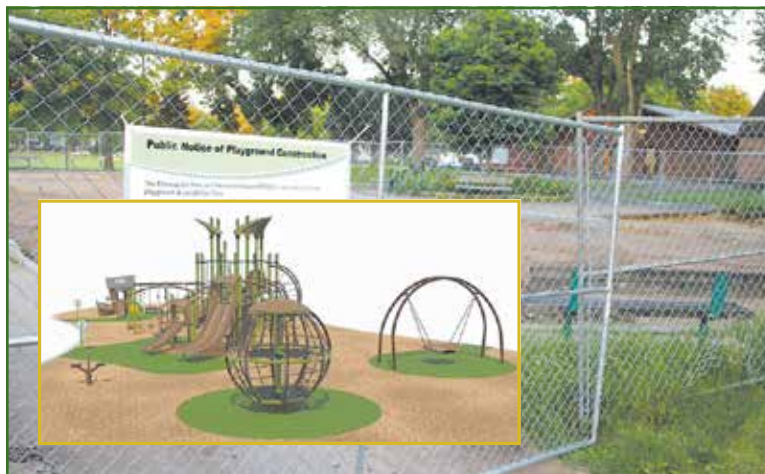
Photo: Work at the site began in June when the old equipment was removed, the site graded, and a fence erected. The pool has remained open during the project. The current playground equipment at Longfellow Park was installed in the late 1980s and had reached the end of its lifespan, according to park board staff. (Photo by Tesha M. Christensen)
