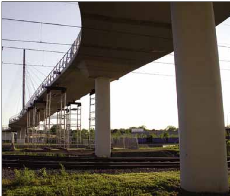
Before the Sabo Bridge is reopened, additional supports will be added. City officials hope to reopen the bridge on June 4. (Photo by Tesha M. Christensen)
