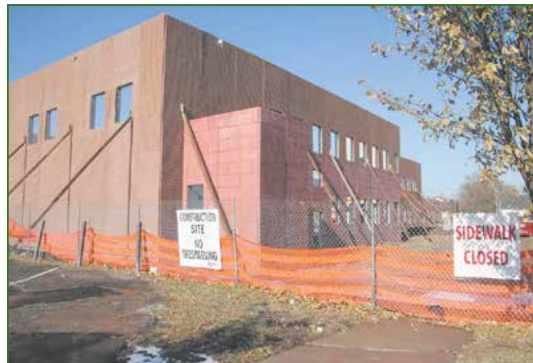
A 19,600-square-foot second-story addition is currently under construction on the back side of the former Rainbow Foods building. When it is complete, Universal Academy Charter School will have 31 classrooms and 55,000 square feet, with an entrance on the east side off 29th Ave. (Photo by Tesha M. Christensen)
