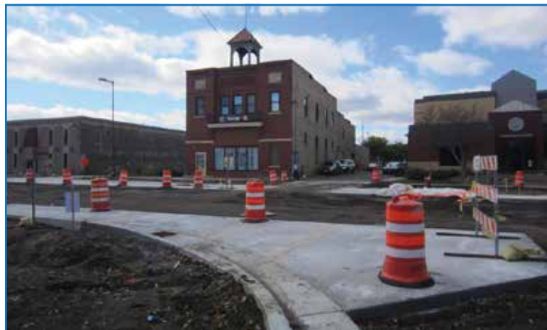
Local businesses felt the impact of road construction over the last couple years. (Photo courtesy of Lake Street Council)
