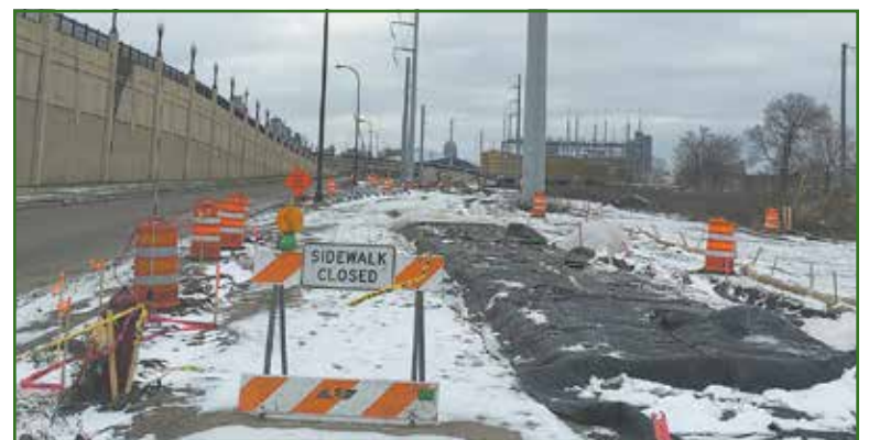
Currently, the first section of Min Hi Line pathway is being installed by the city just south of the bridge between the Greenway and Lake St. "It is very exciting to see the aspiration for the complete Min Hi Line begin to be realized through trail installations at the north and south ends of the corridor," commented Min High Line Coalition co-founder Cora Peterson, who grew up in the Nokomis neighborhood. (Photo by Tesha M. Christensen)
