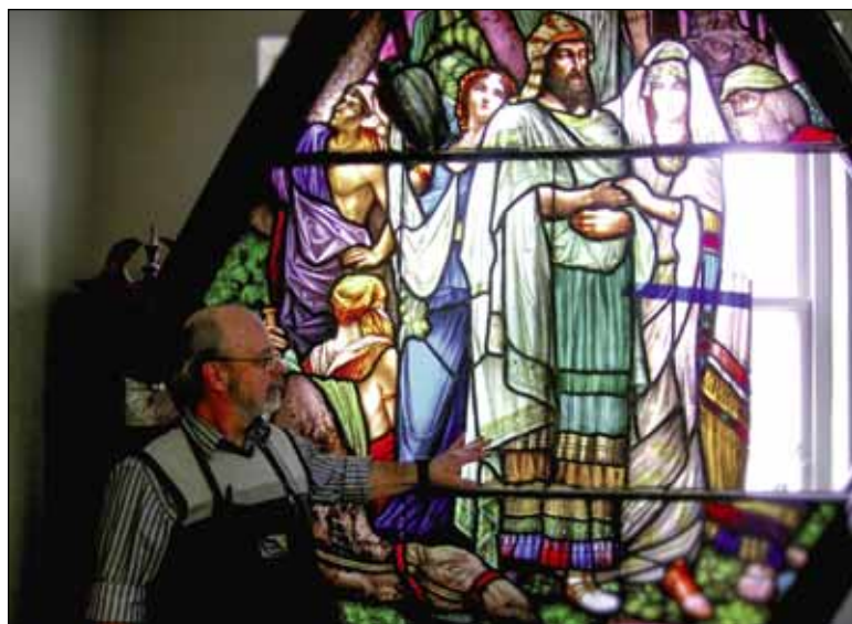
John Sandy at Glass Endeavors talks about a window he is repairing from the 1800s. (Photo by Jan Willms)
