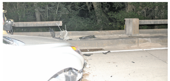
DAMAGE TO BRIDGE
