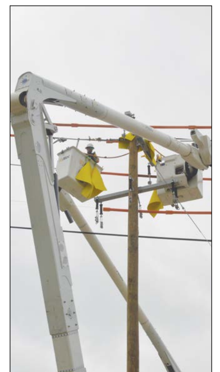
CHRISTOPHER AMOS/THE COMMUNITY NEWS Workers are moving power lines so the old train depot can be moved and construction on the new Aledo City Hall can begin.
