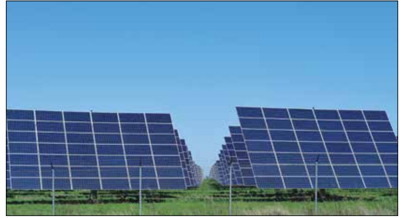
Solar power station near Lake Stamford in north central Texas with lots of blue sky above rows of solar panels.
