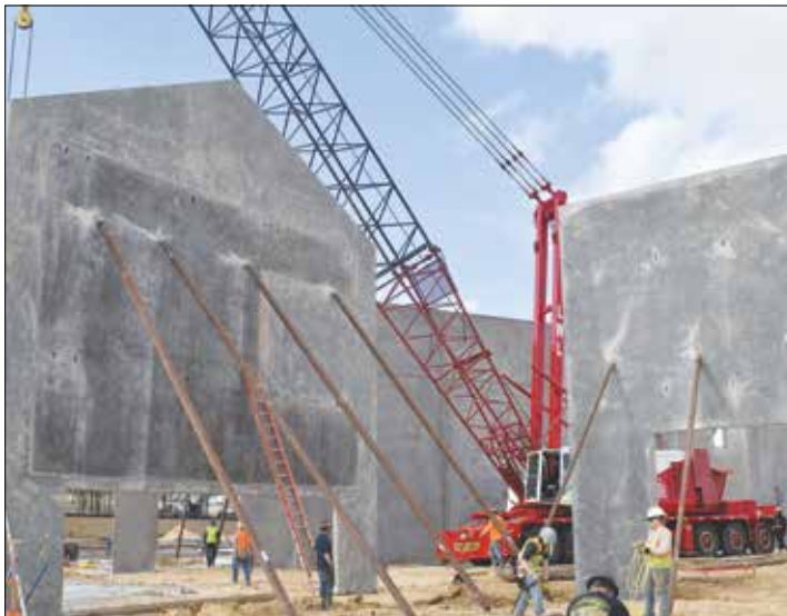
After many months of dirt work, utility installation, and road construction, the new Willow Park Baptist Church started to take shape. From the Feb. 12 issue.
