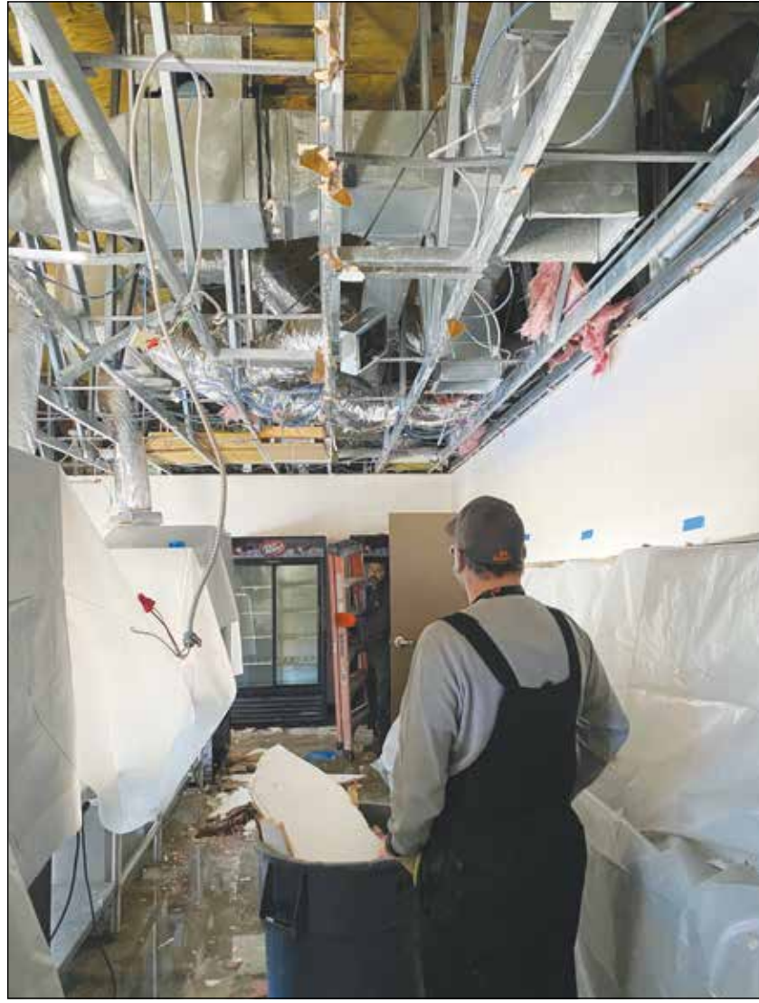
SPECIAL TO THE COMMUNITY NEWS Aledo ISD workers begin cleanup at the Bearcat Stadium concession stand, where burst pipes cause water damage during Winter Storm Uri.
