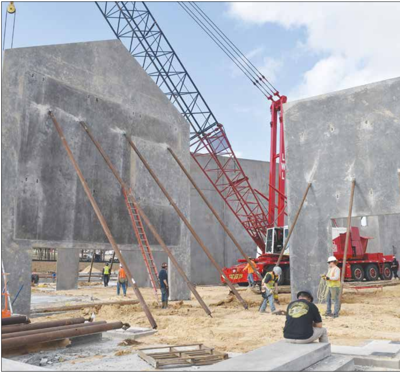
After many months of dirt work, utility installation, and road construction, the new Willow Park Baptist Church has started to take shape at Crown Pointe. The construction of the sanctuary and additional facilities should be ready in early 2022.
